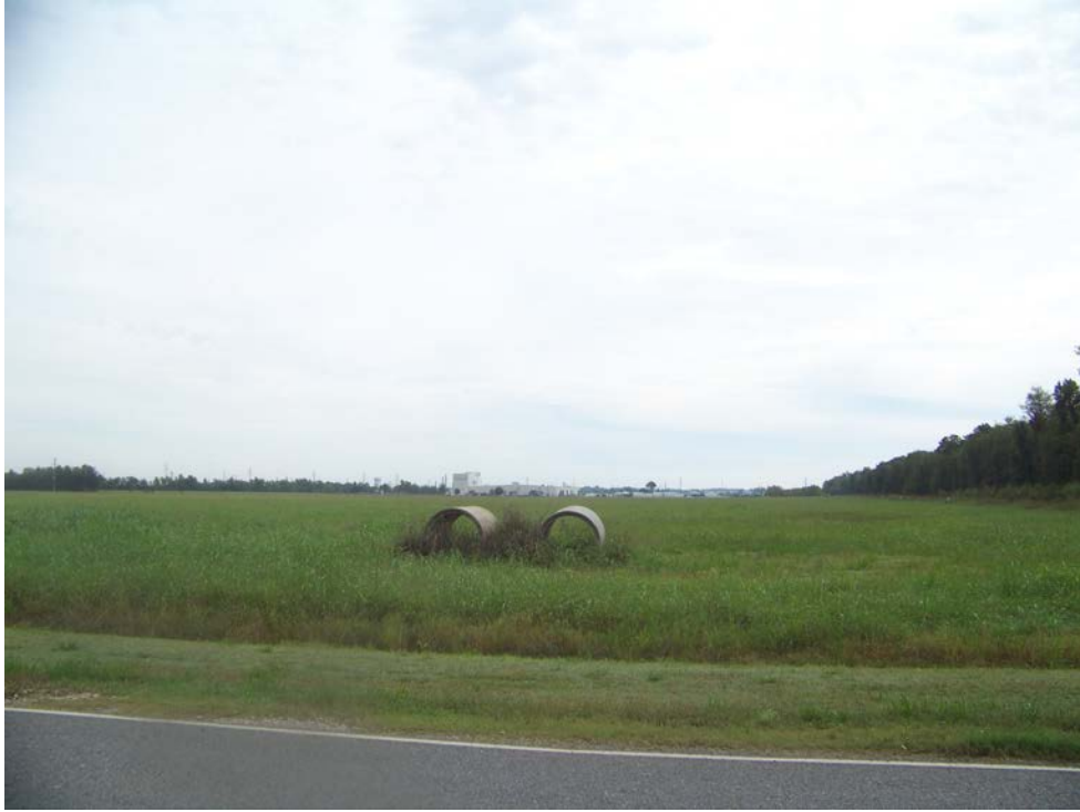
Photograph 6. Two culverts located on the southwestern portion of the property along Enterprise Blvd.
