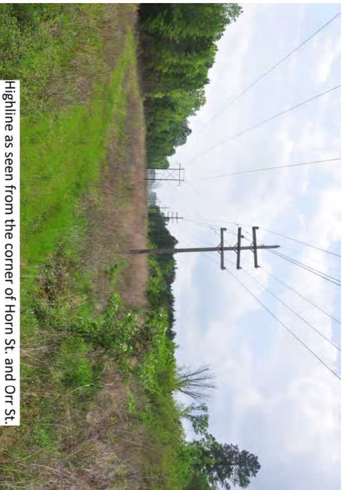
Debris along gas line
