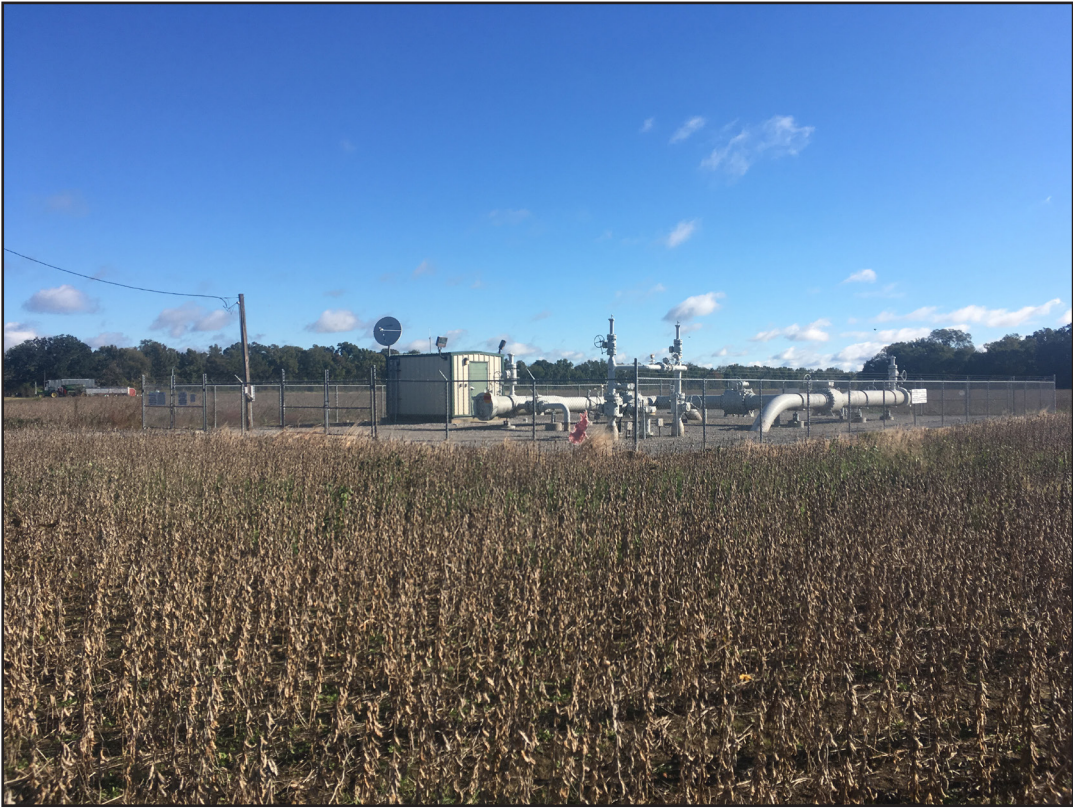
Figure 5.2. View of carbon dioxide station in project area, facing northeast.
