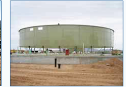
Synchronized jacks are used to erect bolted-panel tanks from the ground up. Workers stay on the ground and perform no hot work which makes tank construction safer compared to field-welded methods.
