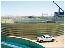
Mechanical components are installed, including blowers, pumps, aeration units, clarifiers, SBR components (when appropriate), grating and plumbing.
