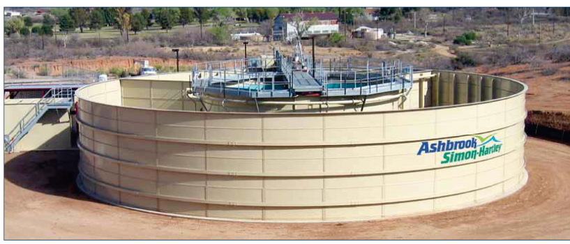
Scope includes: blowers; Wilfey Weber aeration systems; process and clarification tanks; grating, handrails & staircase; pumps and plumbing.
