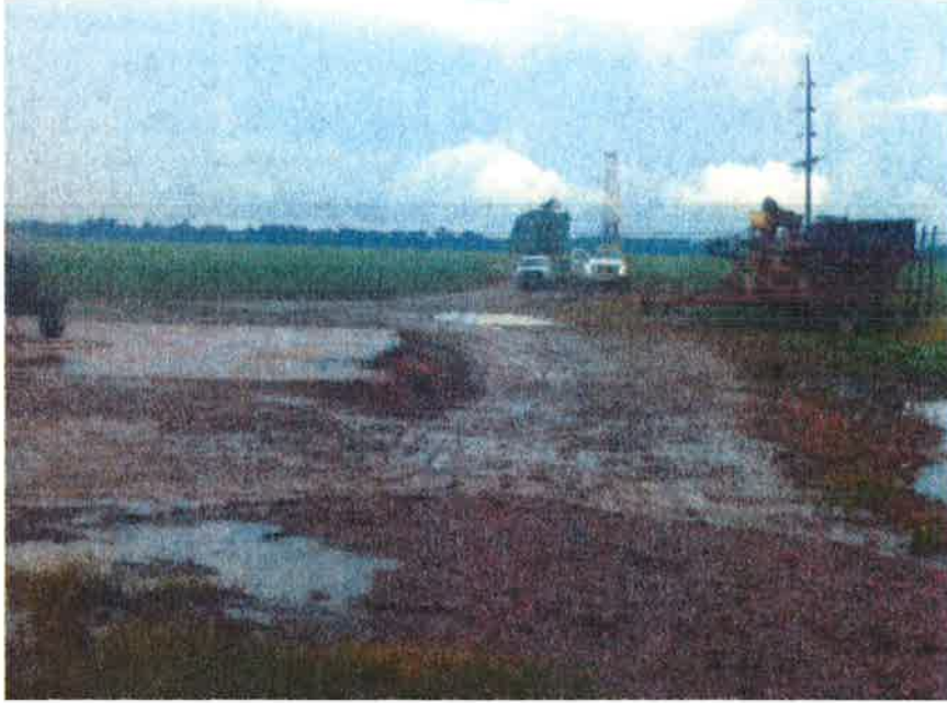
Description: Drill rig and farm equipment on dirt road near concrete slab.
