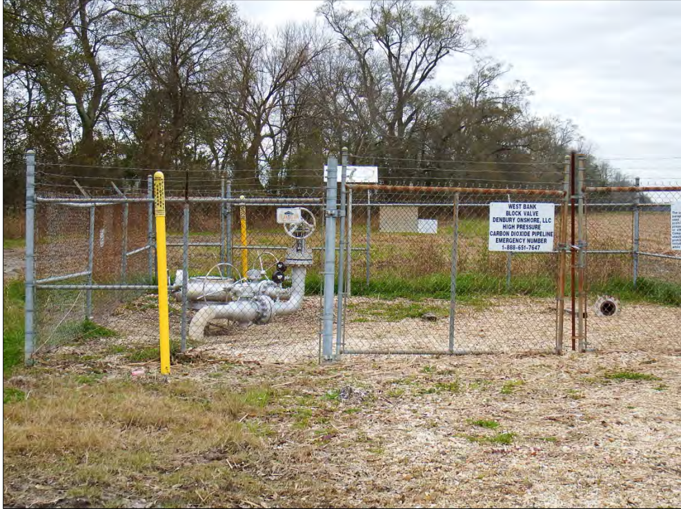
Photograph 21. Carbon Dioxide Pipeline, Northeastern Corner of Property, Facing South
