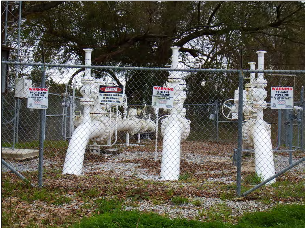
Photograph 20. Propylene and Ethane Pipelines, Northeastern Corner of Property, Facing South
