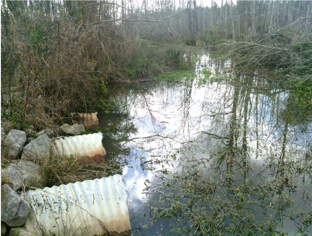
Photograph 95: Six 24-inch culverts from lake to east and canal along eastern boundary.
