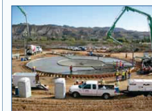
The foundation is prepared and rebar is installed based on foundation plans provided by Ashbrook Simon-Hartley. A working supervisor is also provided to assist with embedded item placement, and to witness the pour.
