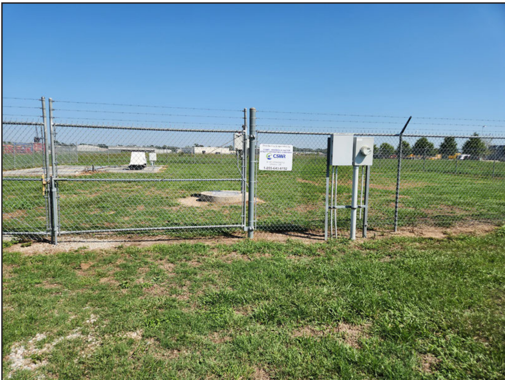
Figure 5.6. View of fenced utility station in the southwest corner, facing north.
