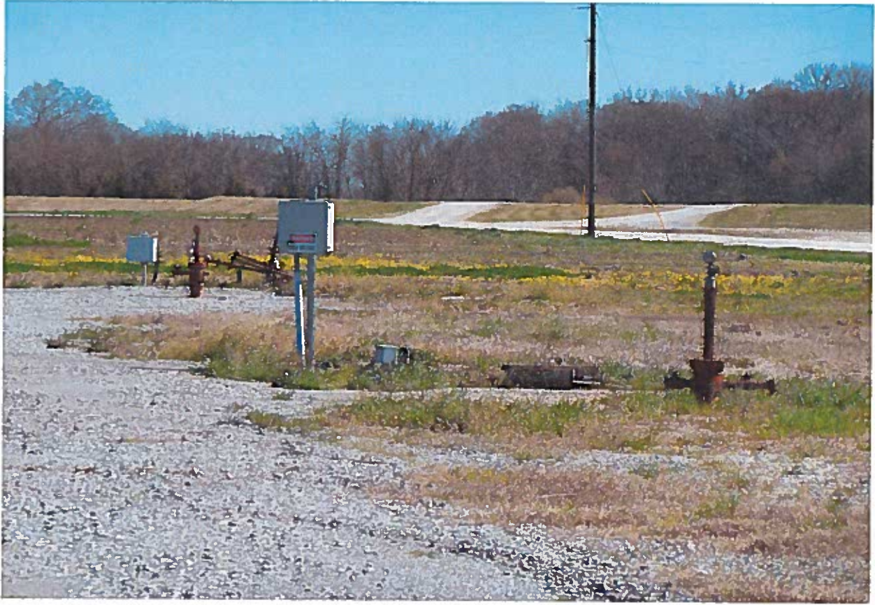
Shut in Gas well site located in the central part of the subject property
