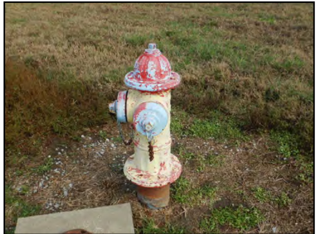
Photo 44: A fire hydrant observed on the central western boundary of the Subject Property.
