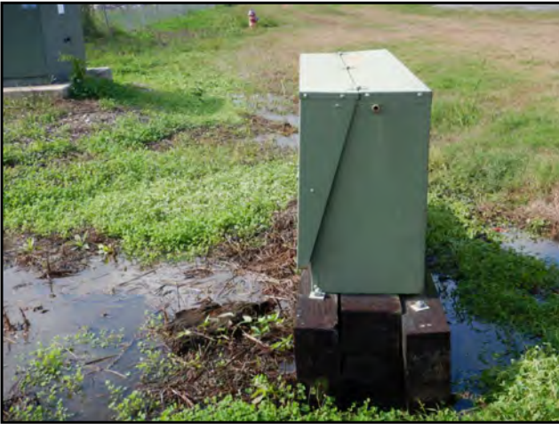
Photo 53: View of a utility vault observed adjacent to the south-southwest of the Subject Property.
