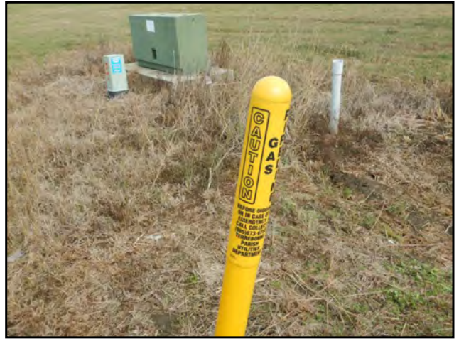
Photo 46: A second parish gas line marker, a cable utility box, and another utility vault observed on the northwestern boundary of the Subject Property.
