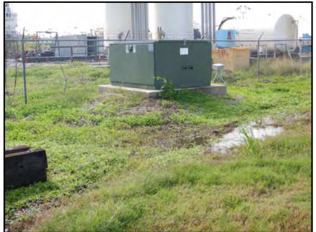
Photo 52: View of a pad mounted transformer observed adjacent to the south-southwest of the Subject Property.
