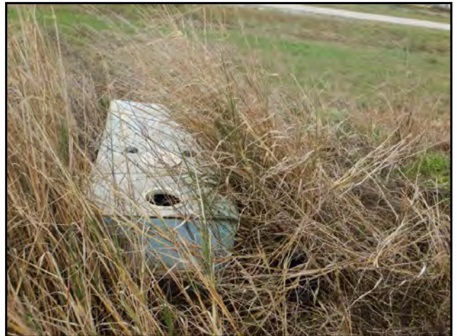
Photo 36: View of a utility vault observed near the southwestern corner of the Subject Property.
