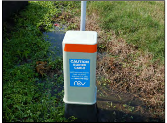
Photo 54: View of a cable marker observed adjacent to the south-southwest of the Subject Property.
