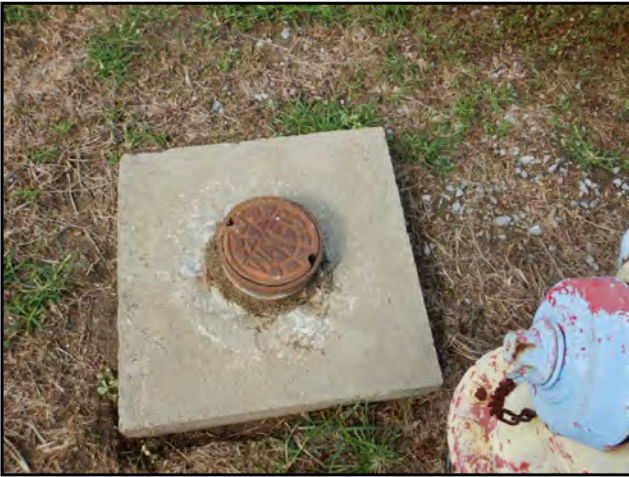
Photo 45: A water utility vault observed on the central western boundary of the Subject Property.
