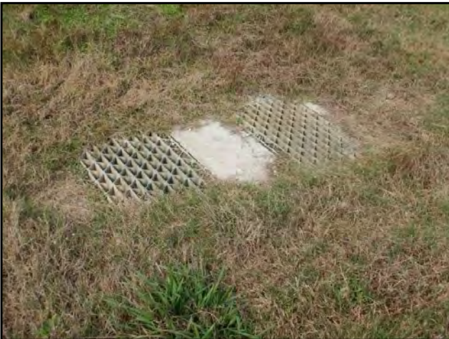
Photo 35: View of a roadside storm drainage basin observed on the southwestern portion of the Subject Property.
