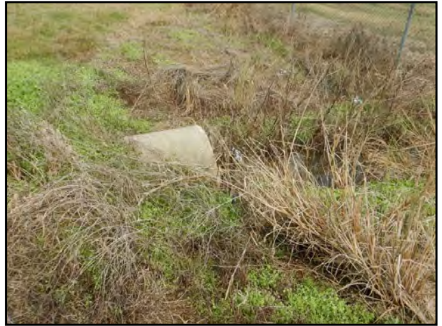
Photo 34: View of the culvert observed along the southwestern boundary of the Subject Property.
