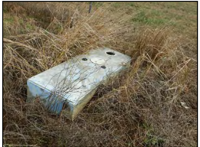
Photo 40: View of a utility vault observed on the southwestern corner of the Subject Property.
