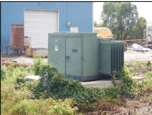
Photo 59: Close up view of the pad mounted transformer observed on the property adjacent to the west-southwest.
