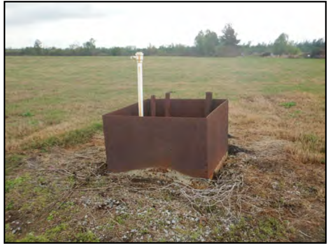
Photo 22: View of a second water source observed on the southern portion of the Subject Property.
