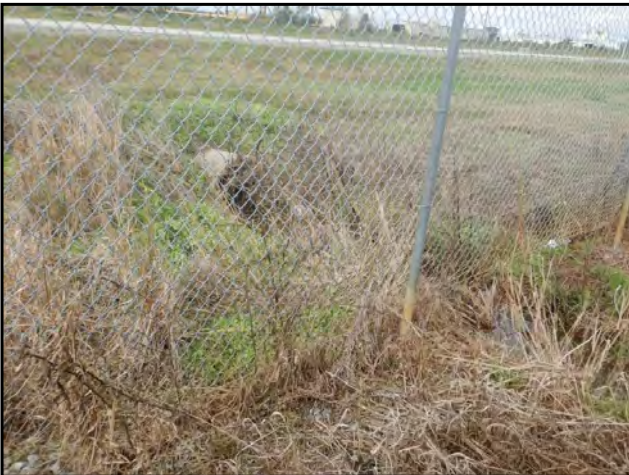
Photo 31: A culvert and ditch observed on the southwestern portion of the Subject Property.
