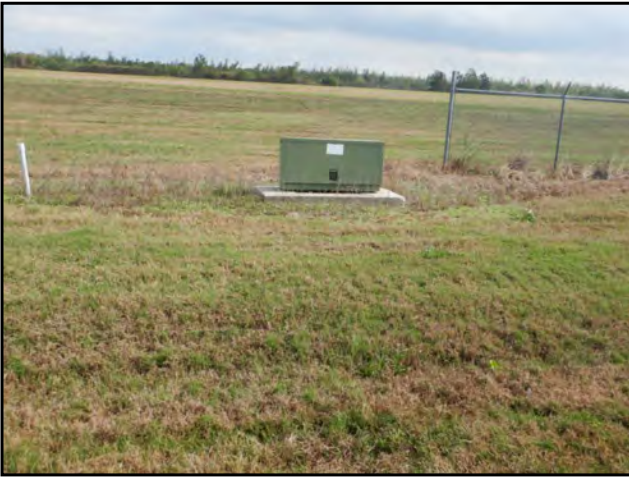
Photo 41: View of a utility vault observed on the central western portion of the Subject Property.
