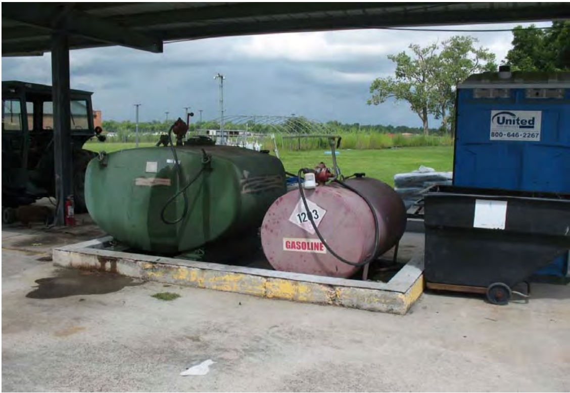
27. View of the gasoline and diesel ASTs located beneath a canopy (Building 3045).
