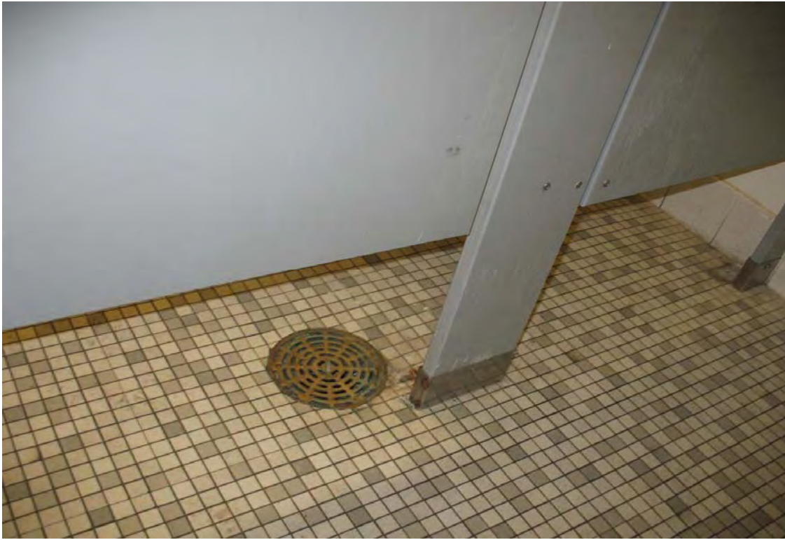
41. View of a floor drain located in one of the bathrooms located in Building 3000.
