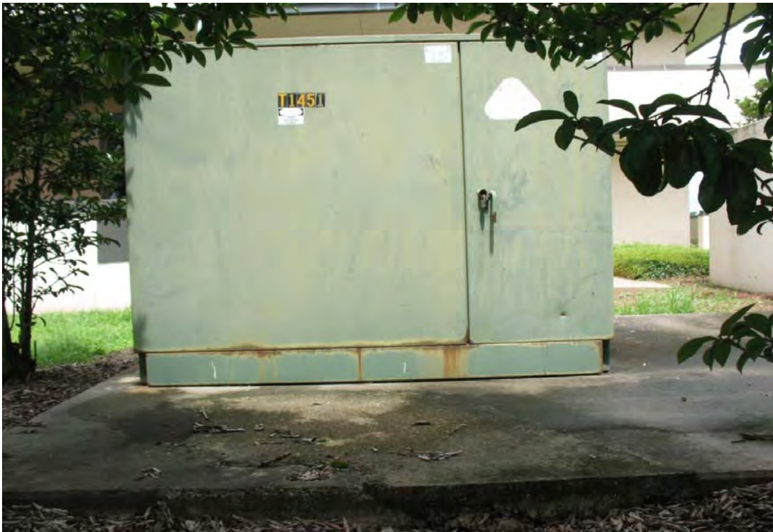
31. View of one of the pad-mounted transformers located at the site. This transformer is located northeast of Building 3100.
