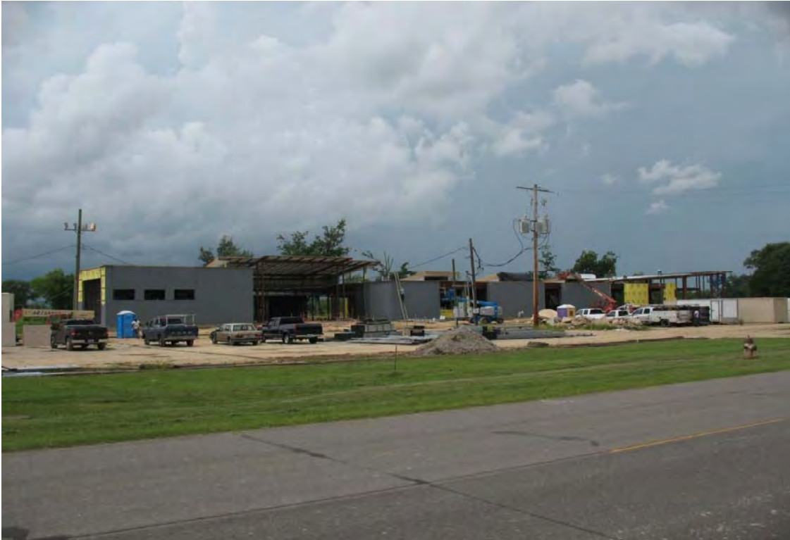
14. Looking south from GSRI Avenue at the building under construction located on the site's northern portion.
