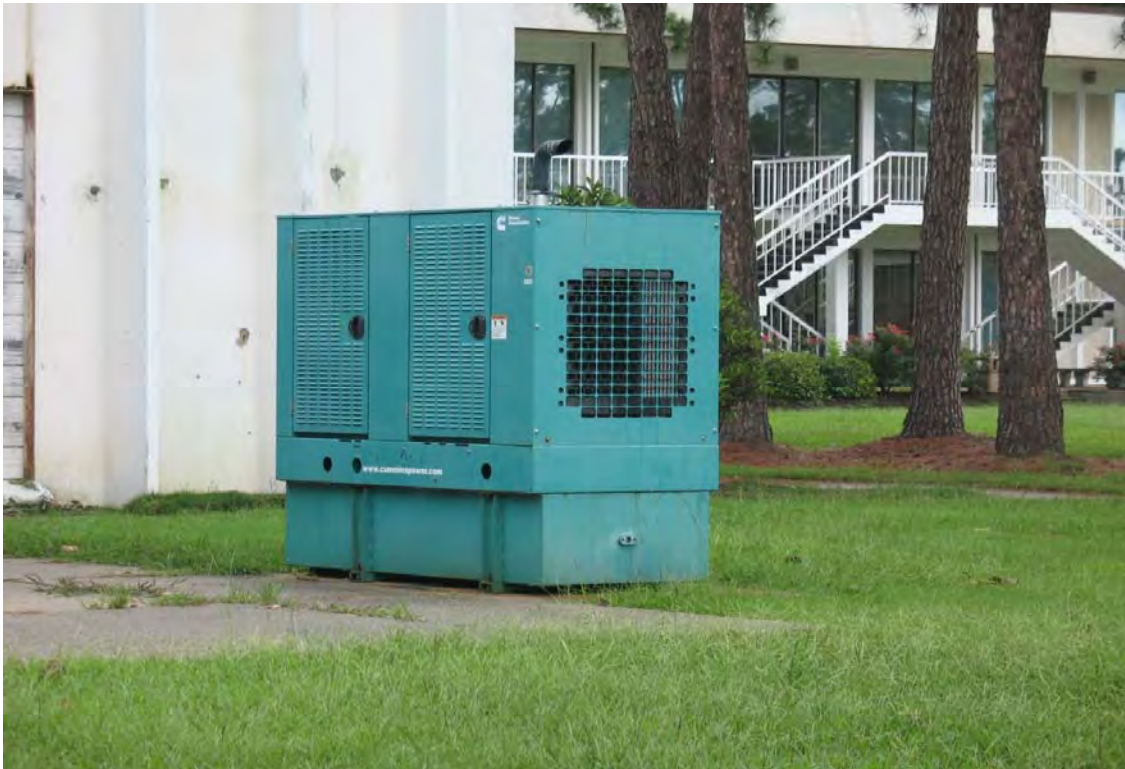
28. View of one of the three emergency generators located at the site. This generator is located south of Building 3110.
