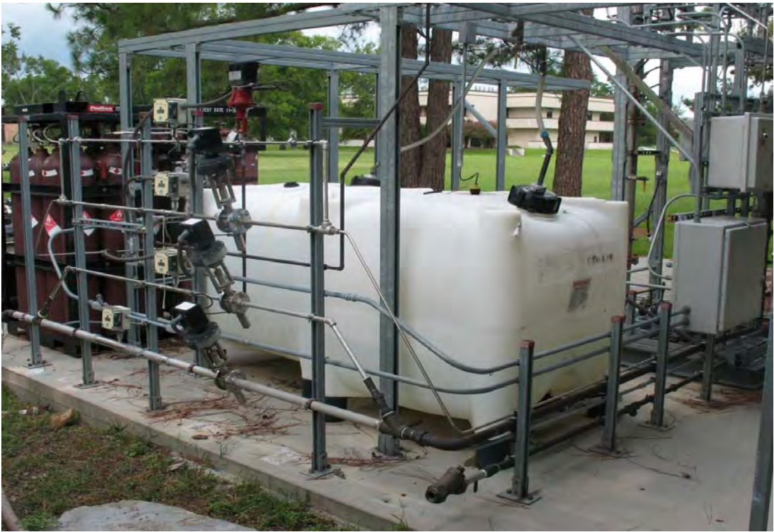
29. View of the totes associated with the Hydro Flame mobile unit located south of Building 3010.
