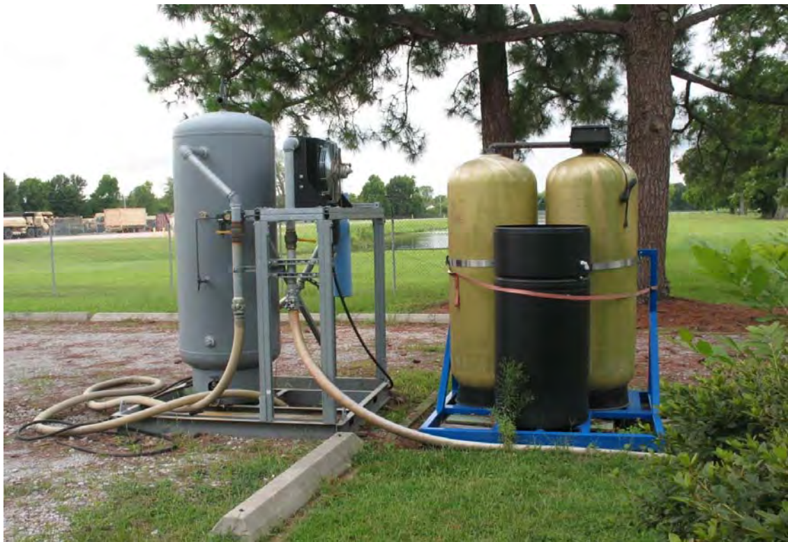
30. View of the tanks associated with the Hydro Flame mobile unit located south of Building 3010.
