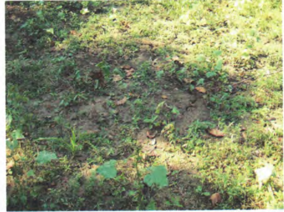
Photograph 8: View of cracked soils in low lying area.
