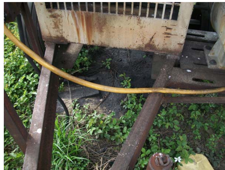
View of soil staining below diesel engine.
