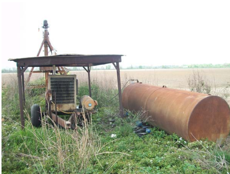
Diesel AST and engine near center of the developed area of the site.
